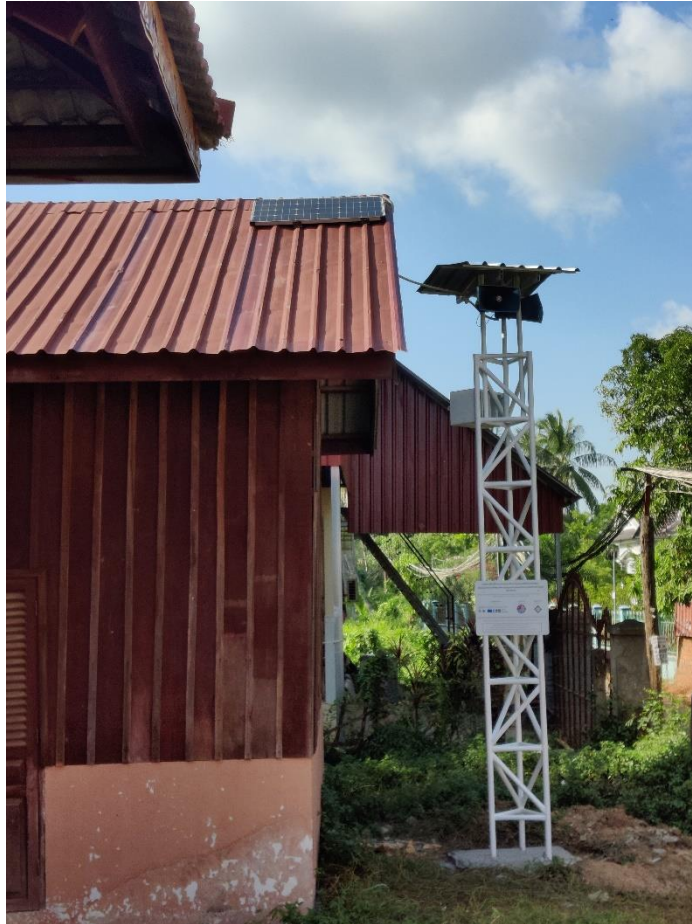
Urban EWS Speaker installed in Kdol Daun Teav Commune, Battambang City, Battambang Province, Cambodia (Photo by People in Need Cambodia).
