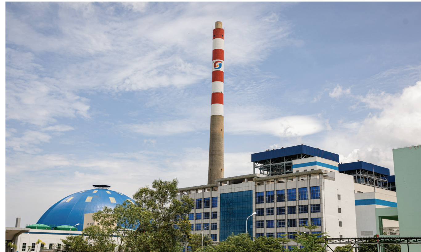
Cambodia's active coal-fired power plants are concentrated in the district of Steung Hav in Sihanoukville province
