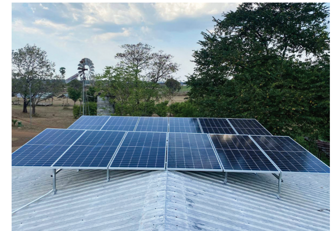
Solar panel in Bateay district, Kampong Cham province (credit to EGE Cambodia Energy Solutions Co., Ltd)
