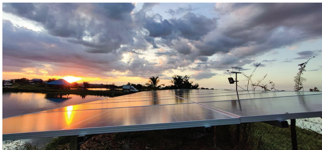
Solar panel in Bateay district, Kampong Cham province (credit to EGE Cambodia Energy Solutions Co., Ltd)
