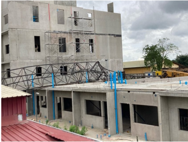
The arm of a crane in Poipet lies horizontal after heavy winds, rain and technical flaws caused the heavy machinery to topple on August 12, 2020. (Ananth Baliga/VOD)
