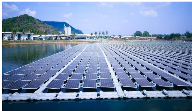
Image: Solar panels in Kampot Source: Property & Construction
