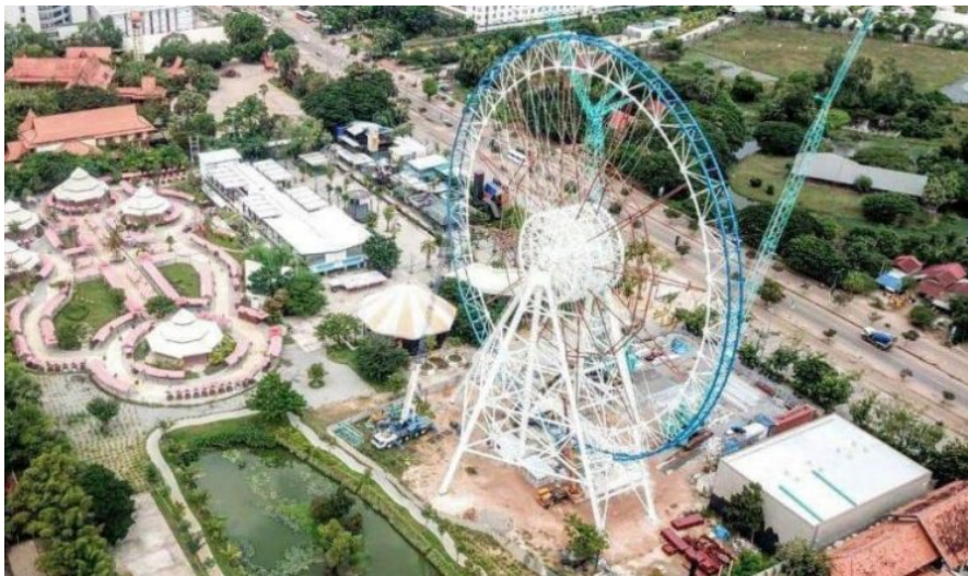
The Angkor Eye taking shape in Siem Reap. Construction and Property Magazine
