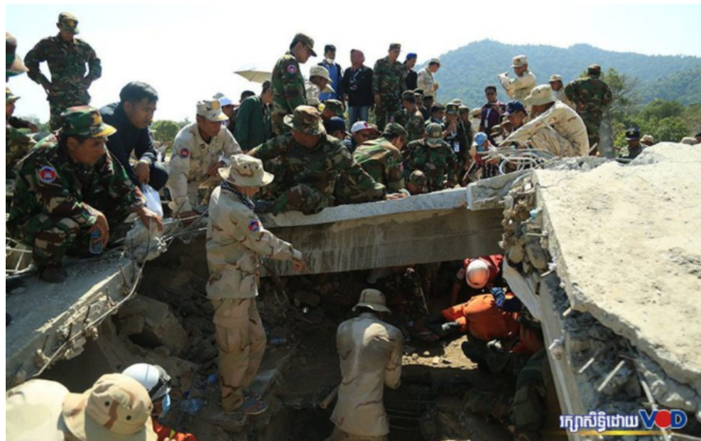
Rescuers search for survivors of a building collapse in Kep province on January 4, 2020. (VOD)
