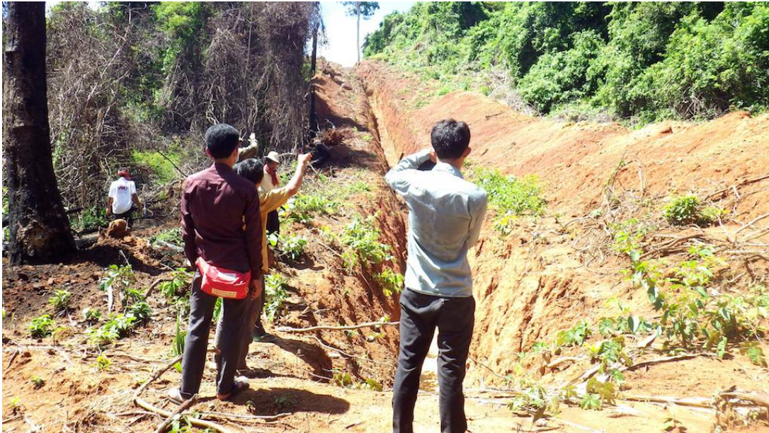
Figure 7. Trench dug by a mining concession company in the forest in Thmea commune
