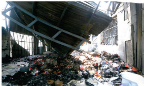
Fire destroys a mattress warehouse in Phnom Penh's Por Senchey district yesterday. KT-Siv Channa
