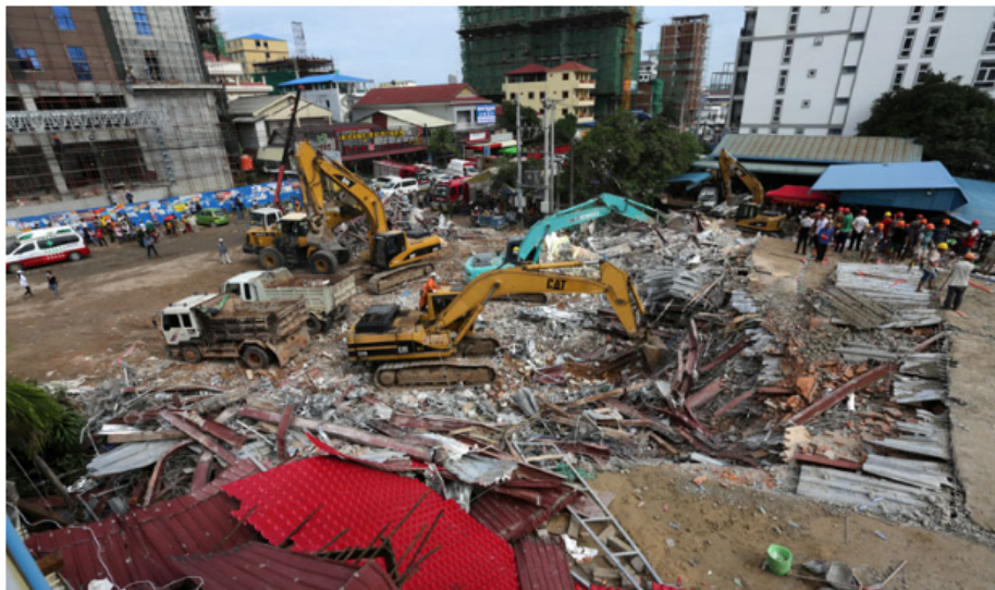
The site of the building collapse in Sihanoukville last year. KT/ Chor Sokuthea
