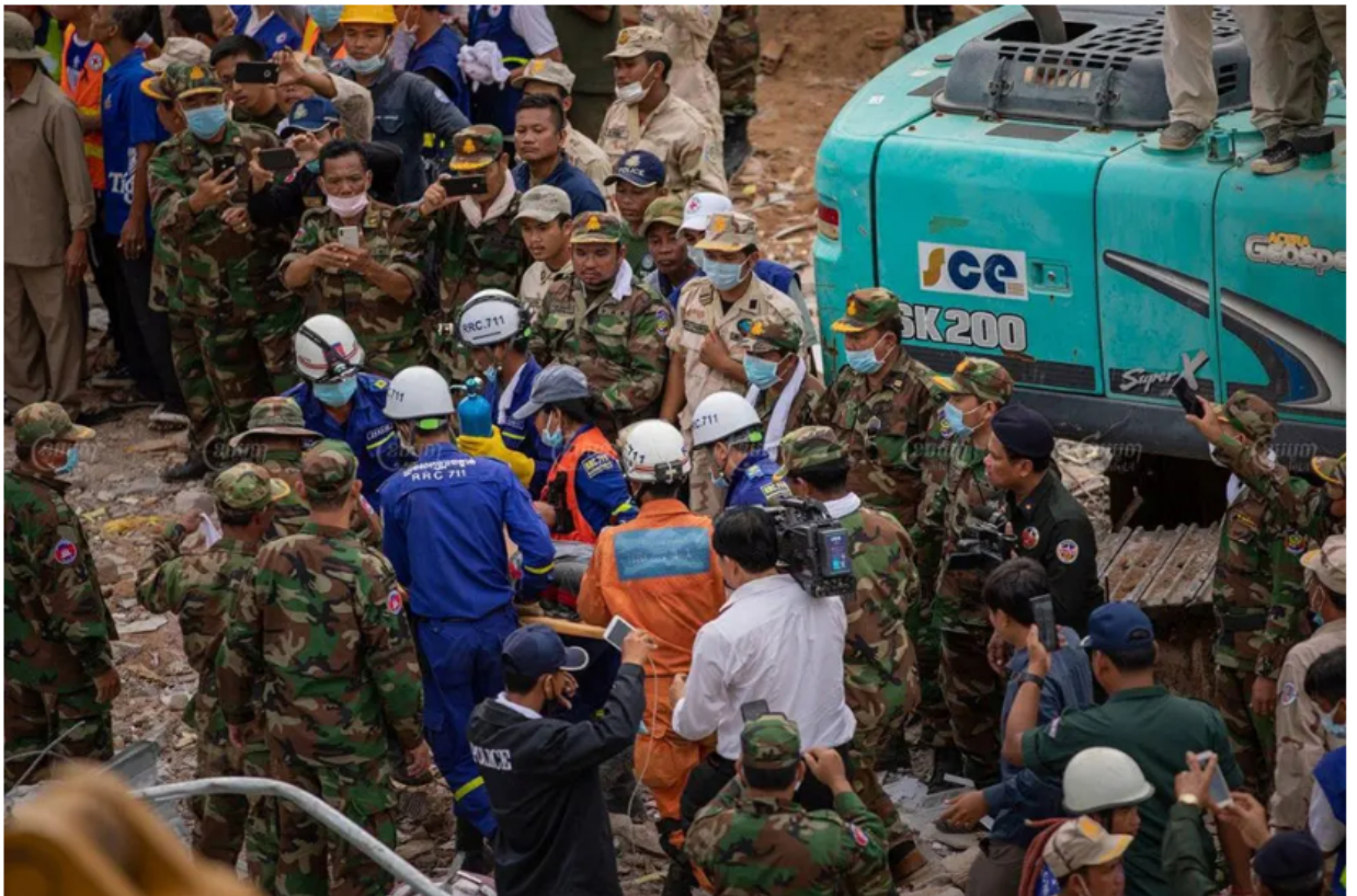
Emergency responders rescue victims of a building collapse in Sihanoukville in June 2019. Central
