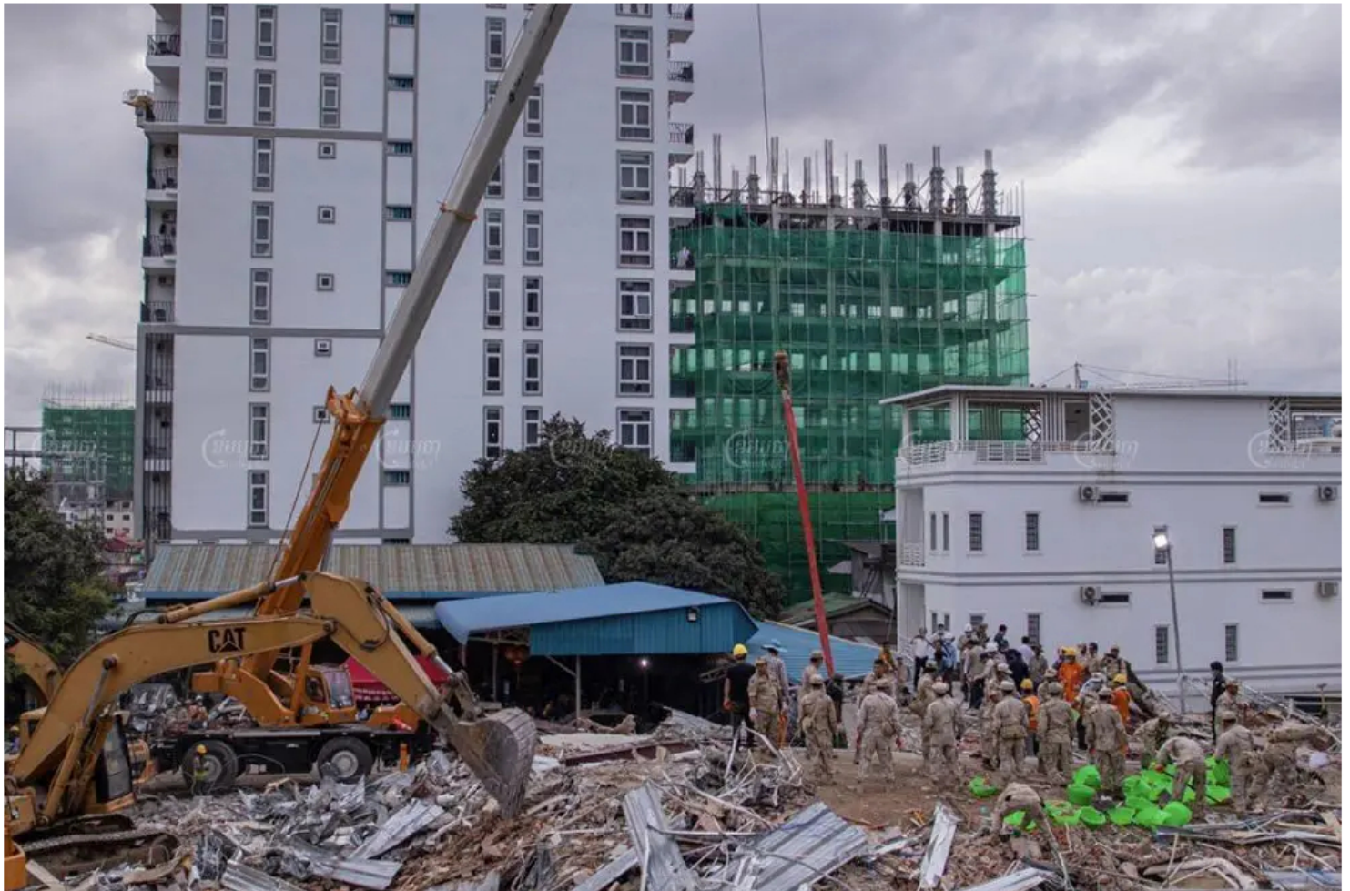
Responders search for victims at the site of a building collapse that killed 28 in Sihanoukville in June 2019. Central
