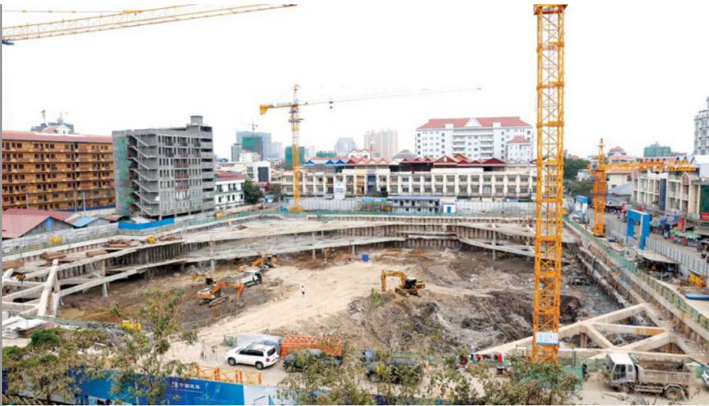
A bird's eye view of the Sino Plaza development shows that construction is still very much active.
