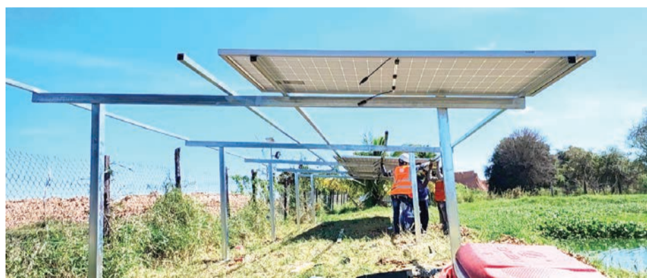
The solar-powered water pump installed by EGE Cambodia. EGE Cambodia
