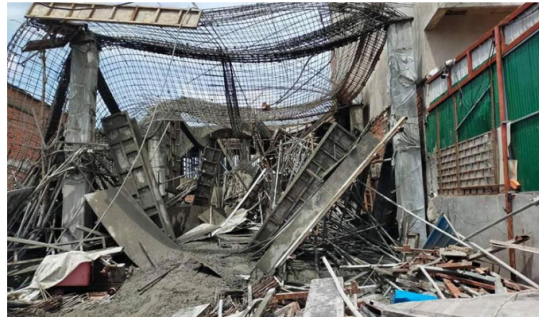
Experts probe cause for building collapse that injured three workers in Banteay Meanchey Province. Facebook
