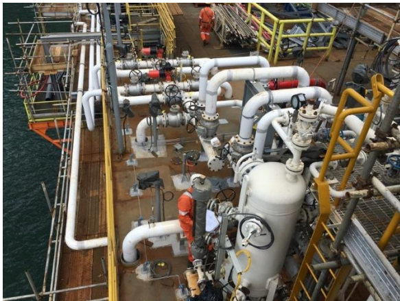
Gas flare scrubber
