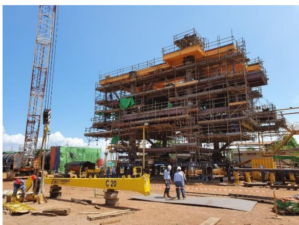
Three decks stacked in the topsides structure of the Mini-Platform
