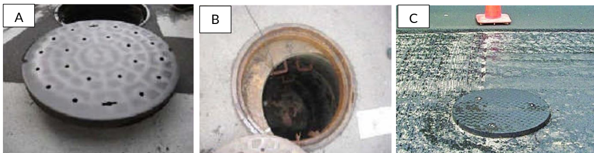
Figure 20. Examples of damages of the manhole, (A) wear of cover, (B) offset of manhole block, and (C) Not coinciding with the height of the road surface
