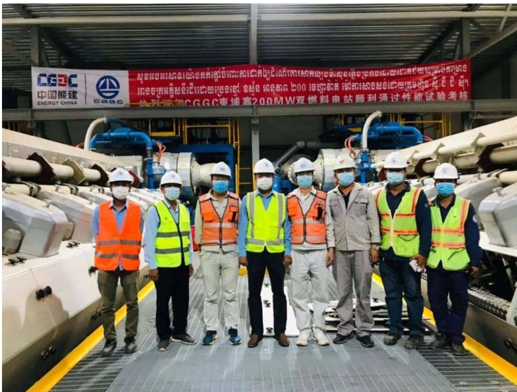
Inside the Gezhouba-built power plant, December 2020. Source: CGGC-UN Power Facebook page .
